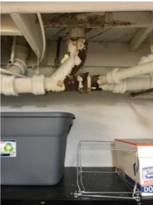
Paint peeling from sewage pipe
