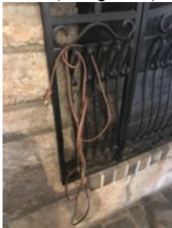
Fire hazard and potential trip hazard
