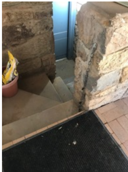
Chains need to be across stairways
