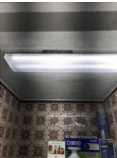
Entry/Exit for mice behind ceiling fixture UPSTAIRS BATHROOM
