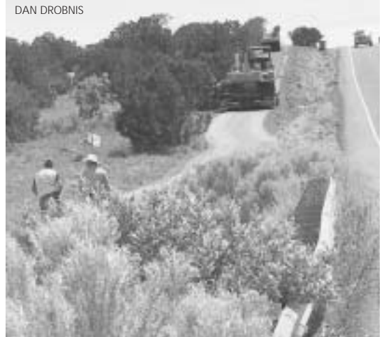
Along the 2.7 mile western hike/bike trail project, every effort was made to spare existing trees. Only about a dozen trees required extensive pruning, and only two were removed completely.
