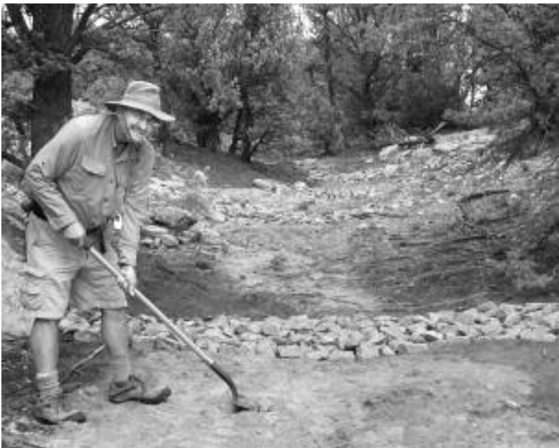
Jim Daniel in front of newly constructed rock dams used to slow water flow. Want to help? See story on p. 4.
